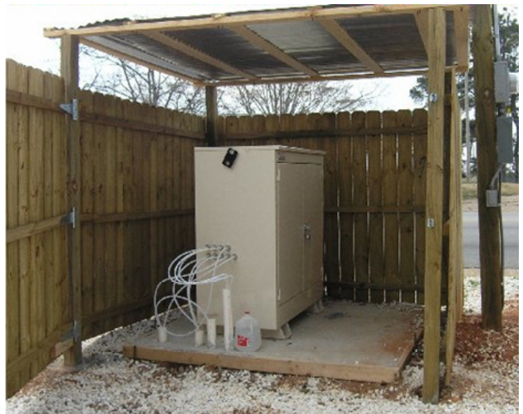
OS-150 on-site in Alabama
