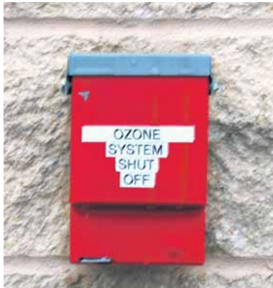
Ozone generator emergency shut-off should be located OUTSIDE the generator room!
