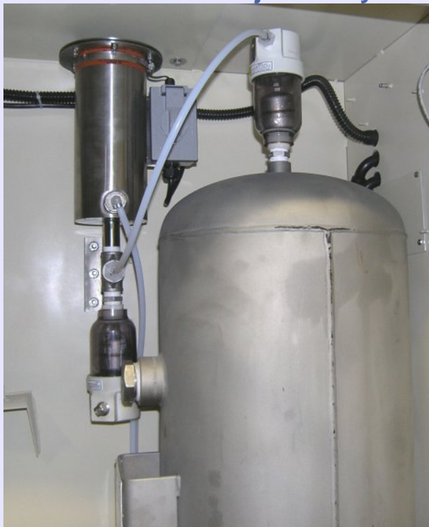
The AVO3 can be used traditionally as an air vent or as a water trap. In this image there is a AVO3 used below the ODS-3H Ozone Destruct Unit to protect it from excess water entering it. To use the AVO3 as a Water Trap the WT-100 can be purchased. This will include the bracket, tee, and all fittings necessary for immediate use at a very reasonable cost.
